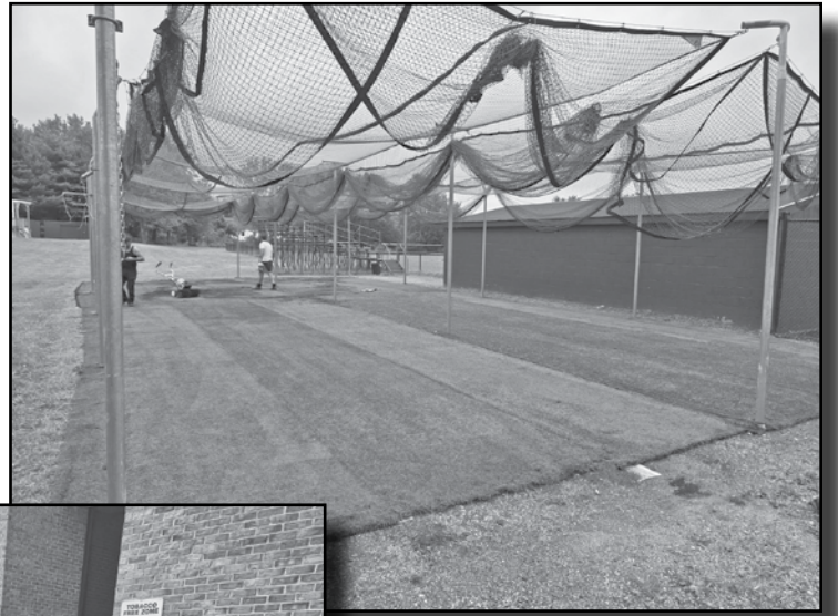
Turf from the old field has been repurposed and placed at the high school batting cages. Also, in preparation for the new track, a drainage system is being installed.
