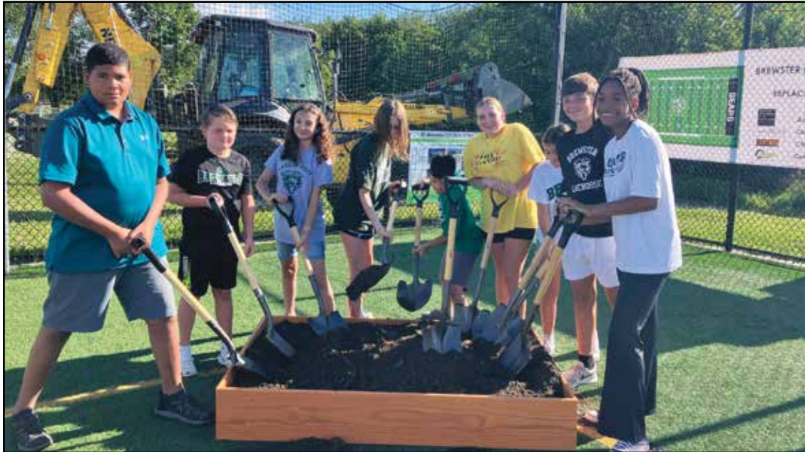
Students helped "break ground" on the Brewster Vision Capital Project on Bears Field recently. Photos courtesy of Brewster Central School District.
