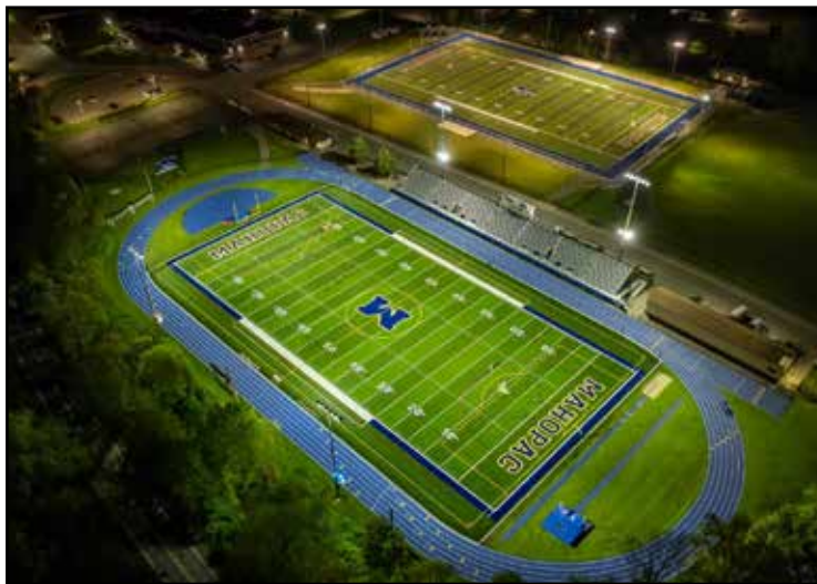
Installation of the new turf field at Mahopac High School was completed during the first phase of the district's capital project.
