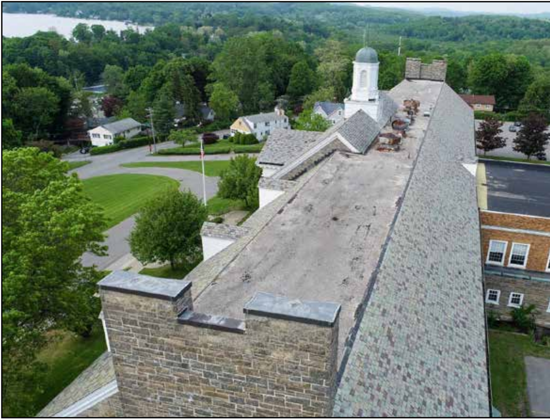
The slate stone roof at Lakeview Elementary School in Mahopac is in need of replacement, and could be done in the summer of 2026 if enough funds are left over from the current capital project. Photos by Tetra Tech Architects & Engineers/The Palombo Group/MCSD.
