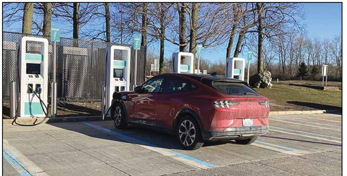
The state is looking to use federal funding to install more electric vehicle fast chargers along major roadways across New York. Photo courtesy of www.thruway.ny.gov .
