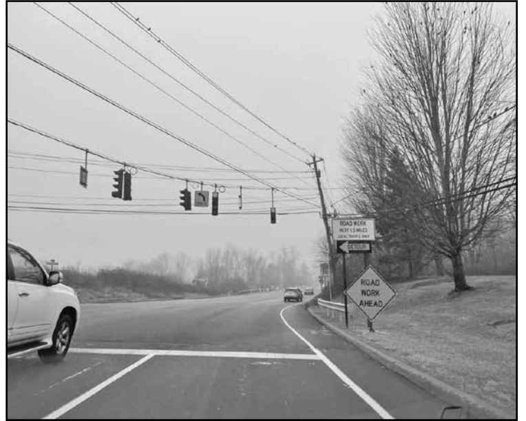
Carmel school administrators and county officials are asking drivers to be cautious when navigating the construction on Fair Street, which is expected to continue through the summer of 2026.
